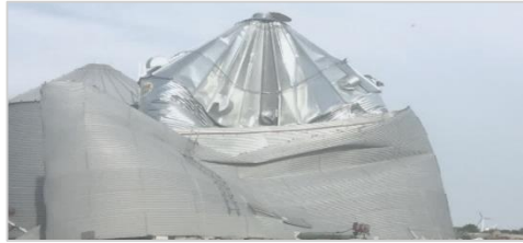
1 Storm damage to grain elevator, Minnesota USA 2017
