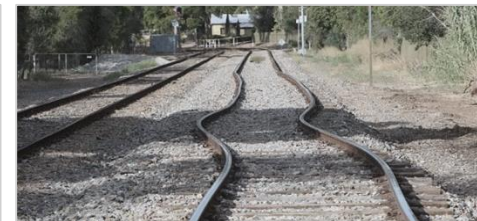
6 Railway heatwave damage, Australia 2015
